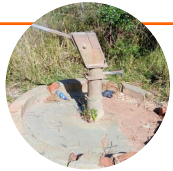
(A non-functional borehole in Luwero, before rehabilitation. Photo submitted by Beatrice Nabukalu )
